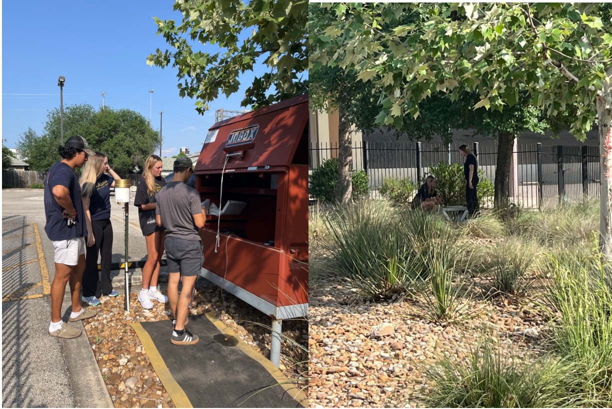
Figure 20 (Left): Sampler Bleeder Controller Installation and Testing. Figure 21 (Right): Testing of Purge Time at the ends of the Bubbler lines.
